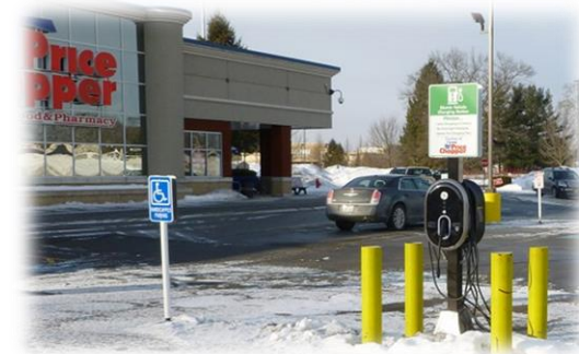
EV Charging Station at Price Chopper Plaza
