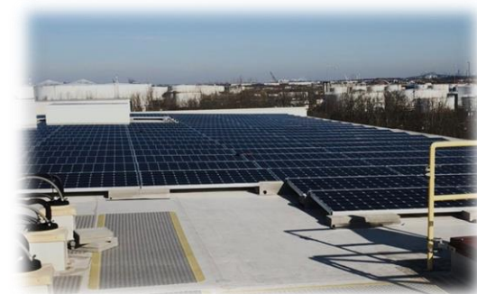
Solar Panel at Carteret Self-Storage
