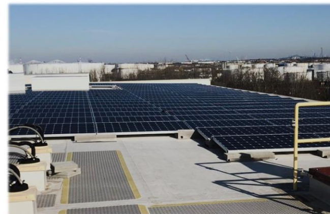
Solar Panel at Carteret Self-Storage
