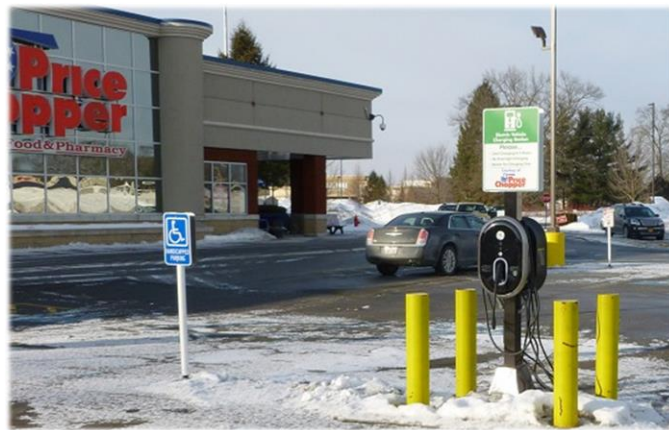
EV Charging Station at Price Chopper Plaza
