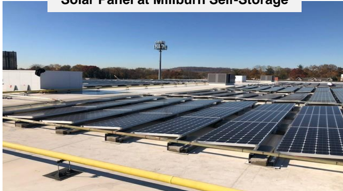
Solar Panel at Millburn Self-Storage
